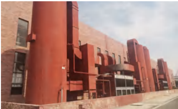
NMP Recovery Unit of Nanjing Gotion
